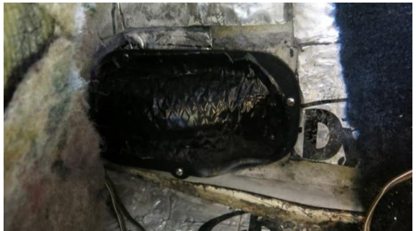
Clark Cover Installed
